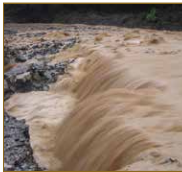
Unmaintained culverts can lead to streams overtaking roads. Photo by Will Harling.
